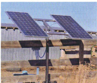
Solar panels capture the sunshine and convert it to DC electricity.
