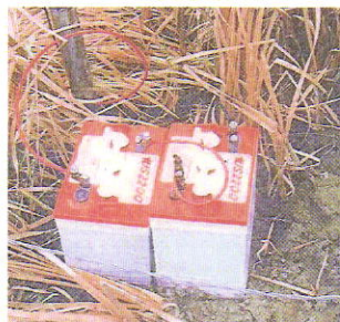
The batteries store the energy.
